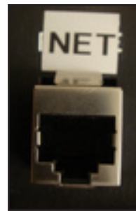
Network Connection on Laptop Plate
